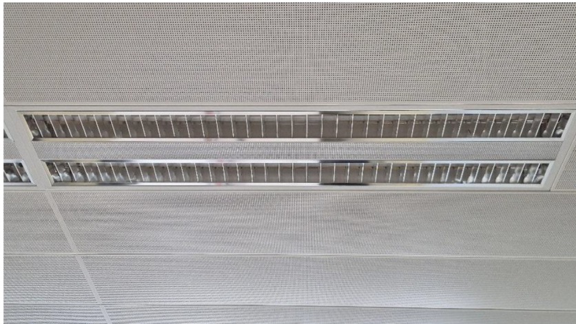
Fig. 2. Recessed luminaire with fluorescent lamp in room 518.
